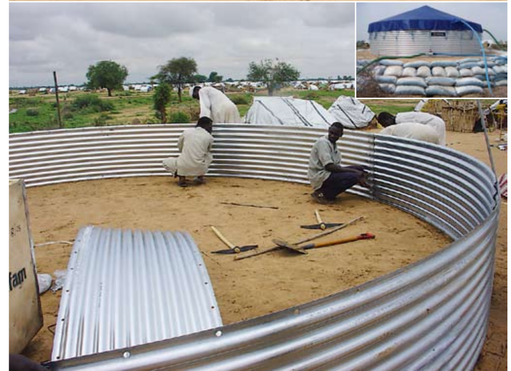
ABOVE: Sudanese refugees, Riyad refugee camp, Darfur, Sudan. BELOW: An Oxfam T70 water tank under construction.
